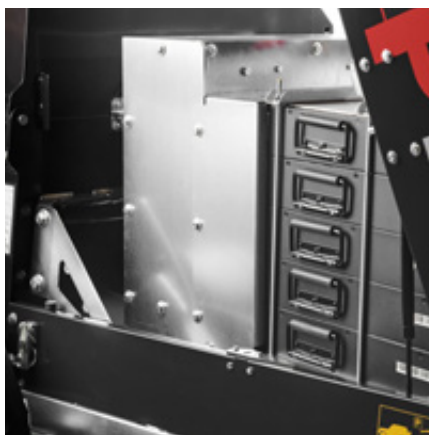
21 kWh. Litiumbatterier (Li-ion, 65VDC, NMC)
