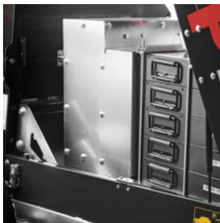
21 kWh Lithium batterier (Li-ion, 65VDC, NMC)
